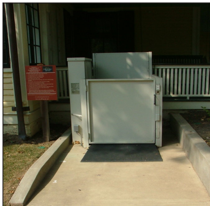
The wheelchair lift provides access to the home's porch and first floor.
